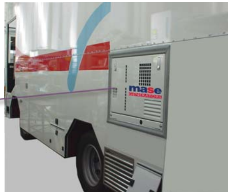
Gen set for telecommunications
